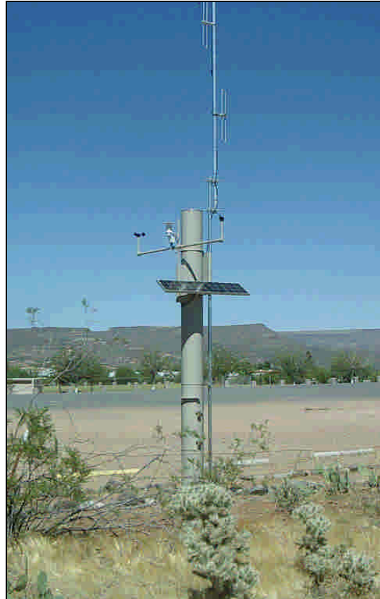
Satellite Repeater Data Concentrator Station, Yavapai County, AZ
